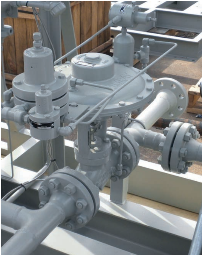
Back pressure control valve.
